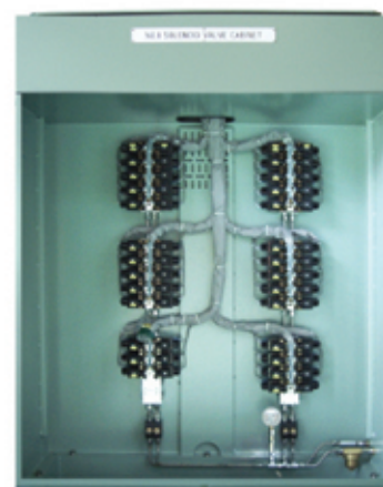
Solenoid Valve Cabinet
